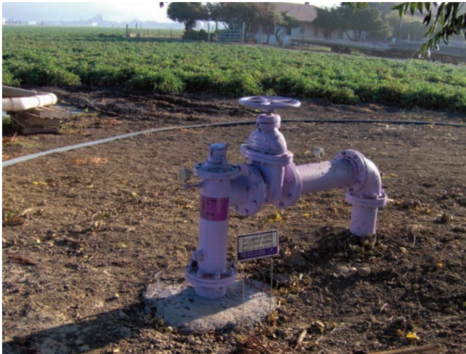
Highly treated recycled water from the Hollister wastewater treatment plant will be used for irrigation of crops once construction of a distribution system is completed.
