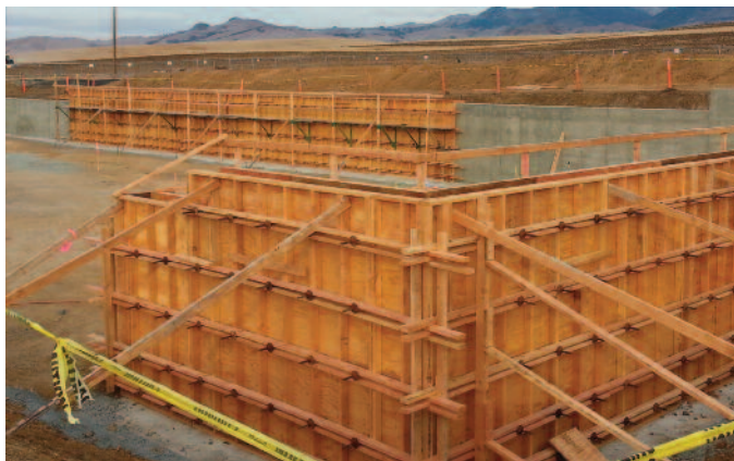
Construction is under way on the upgrade of the Lessalt Water Treatment Plant.
